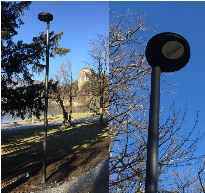
Figure 5: new luminaires with sensors&controllers (Park Vila Zora)
