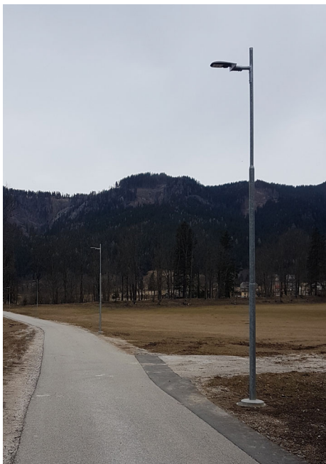
Figure 7: new luminaires on combined poles in Jezersko
